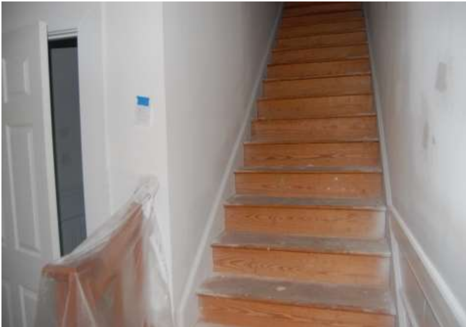
Plate 72. Heywood-Killough House, Interior, New Staircase Installed at the Rear of Original Center Hall.
