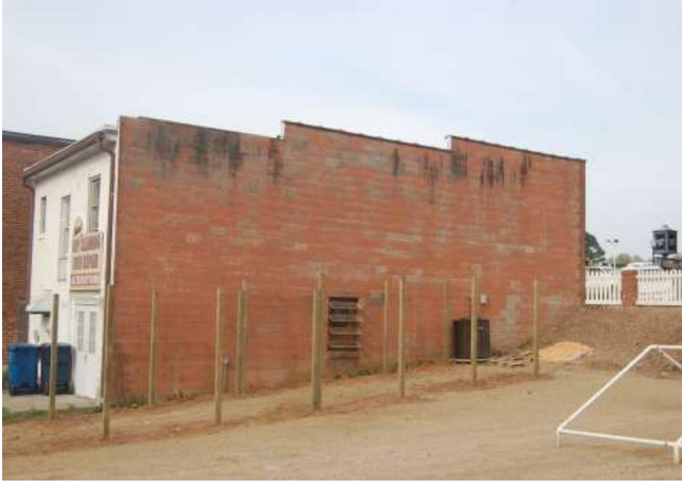
Plate 10. Matthews Commercial Historic District, Proposed Expansion, 1957 Commercial Building at 106 North Trade Street, Side (North) Elevation, Looking Southwest.
