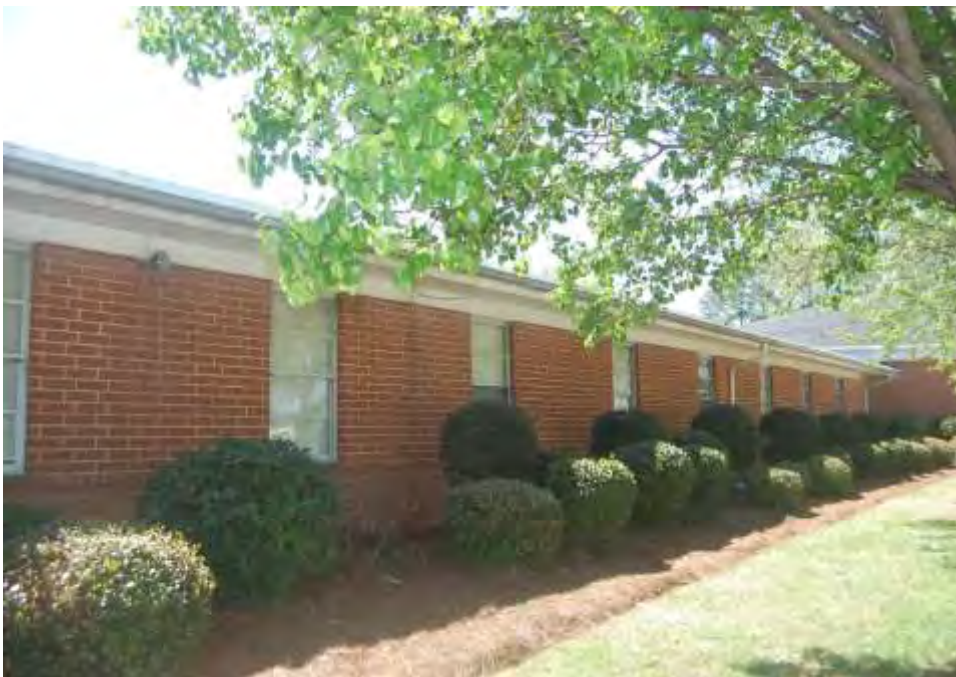
Plate 45. Sun Valley High School, East Classroom Wing, North Elevation, Modern Brick Infill, Looking Southwest.
