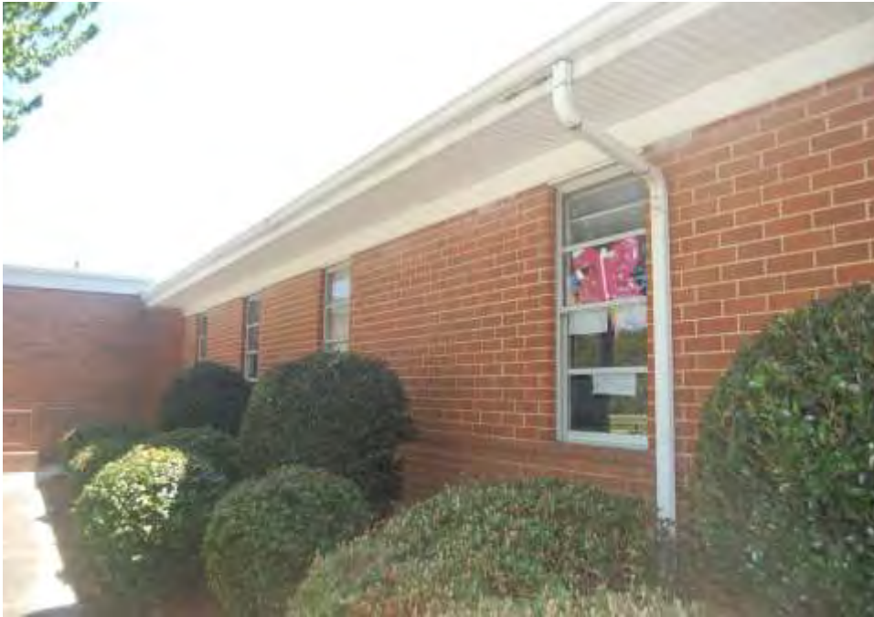
Plate 44. Sun Valley High School, East Classroom Wing, North Elevation, Modern Brick Infill, Looking Southeast.
